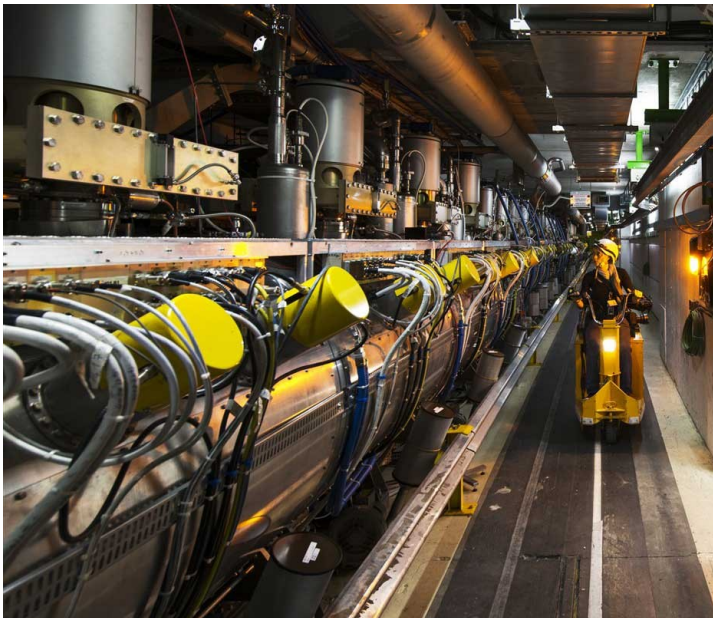
RF cavities at LHC
